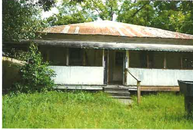
Vacant Home on Baldwin Street ( Below - Evidence of fire damage)
